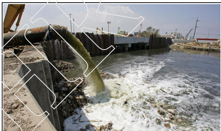
Such means of disposing caused large scale pollution.
